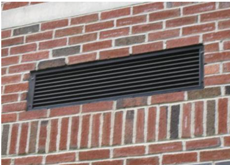
Univent Fresh Air Intake on Exterior Wall
