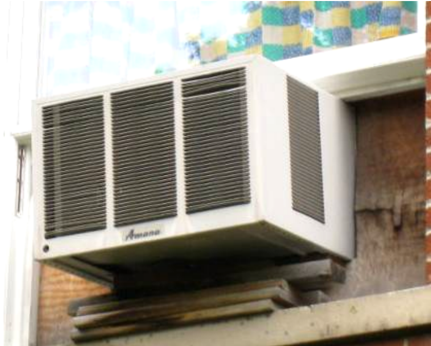
Air Conditioner in Window
