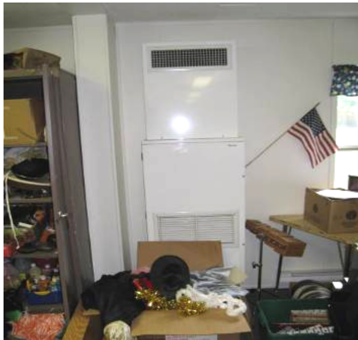
Air Handling Unit on Wall in Modular Classroom Air Diffuser at Top, Exhaust Vent at Base
