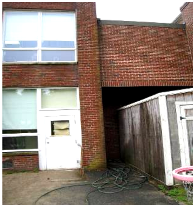
Water Stains on Exterior Brick and Storage Shed
