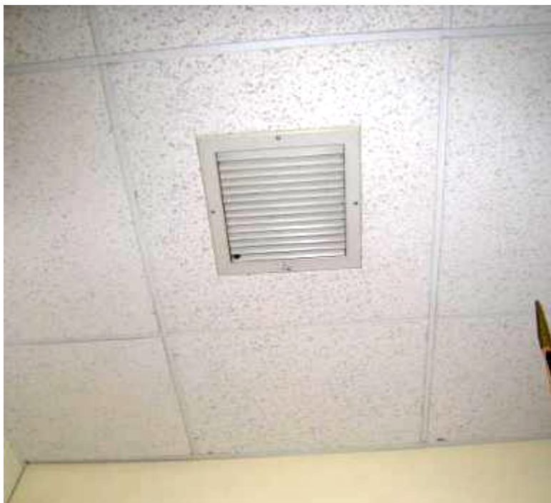
Exhaust Vent on Ceiling
