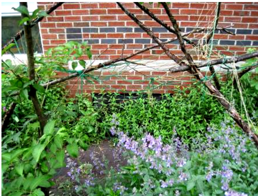
Plants Growing in Front of Fresh Air Intake
