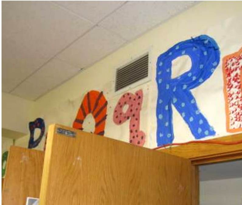
Exhaust Vent on Wall
