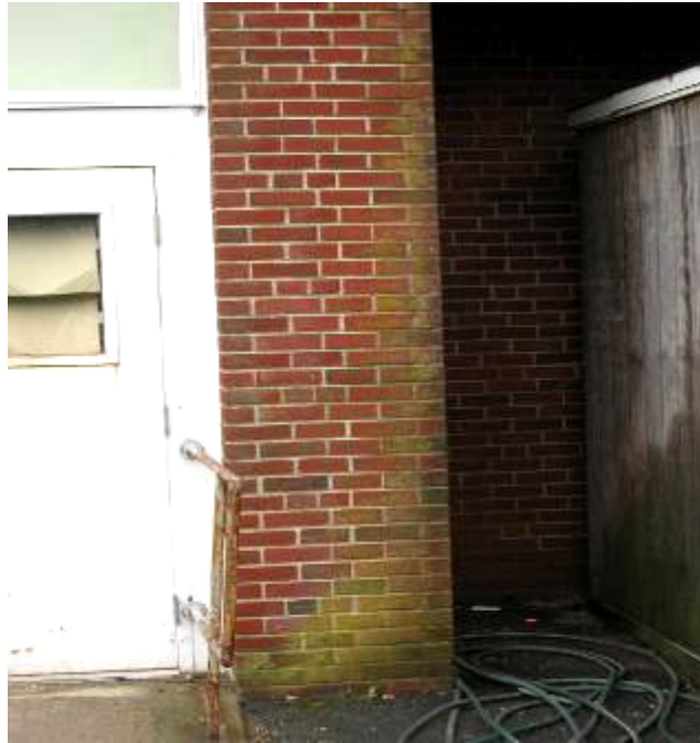
Water Stains on Exterior Brick
