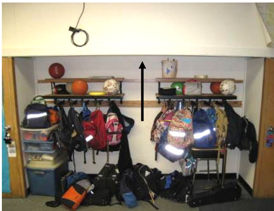
Exhaust Vent in Storage Closet
