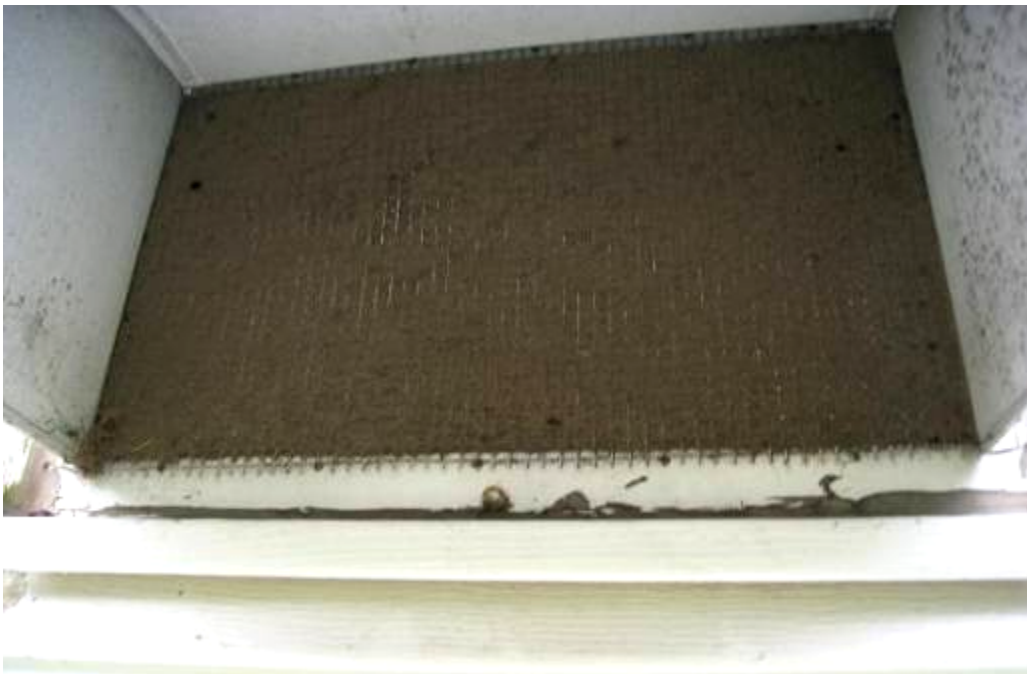
Accumulated Dust and Debris on Air Intake
