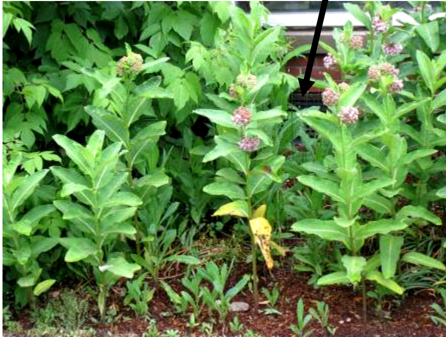
Plants and Shrubs Growing in Front of Fresh Air Intake
