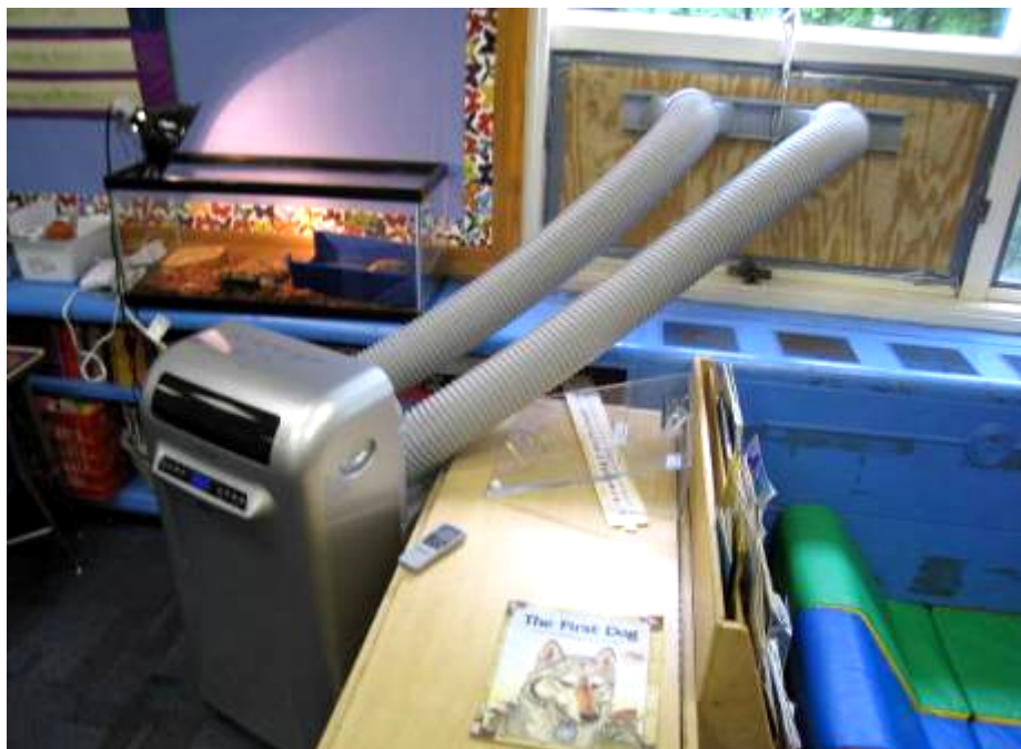
Air Conditioner Ducted to Window by Hoses
