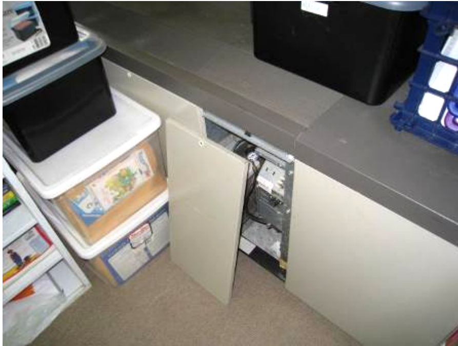
Stored Items on Top and in Front of Univent, Note Panel Removed
