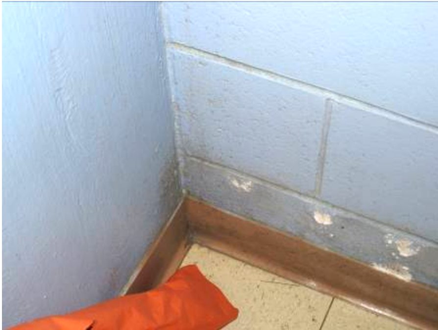
Staining/dirt on wall in teachers' room closet
