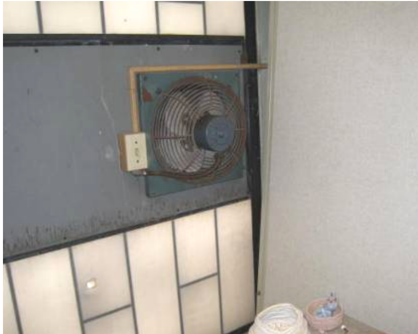
Kiln room exhaust fan with switch
