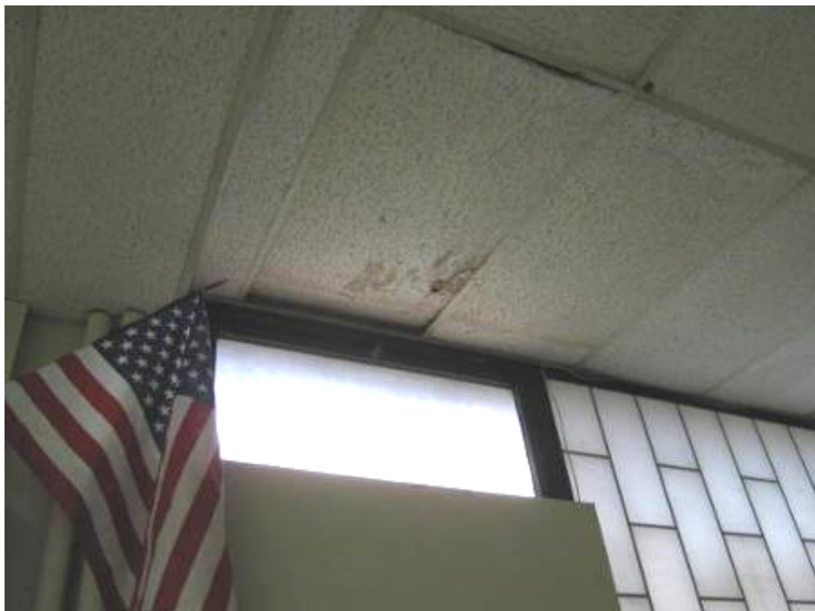
Water-damaged ceiling tiles in room 6A
