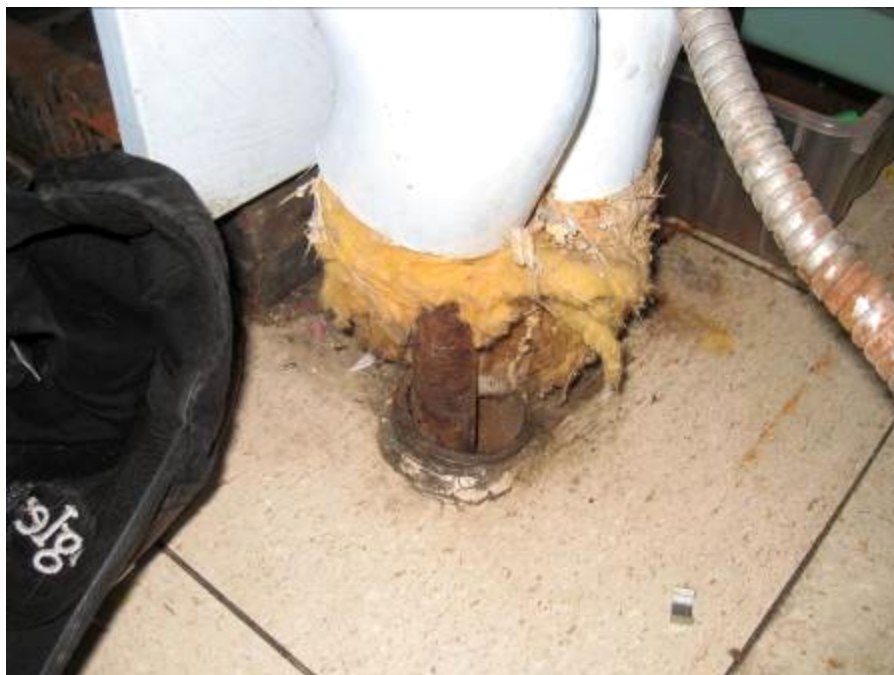
Exposed fiberglass pipe insulation
