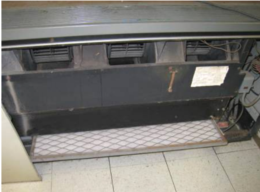
Open univent showing filter material in lattice “cage”
