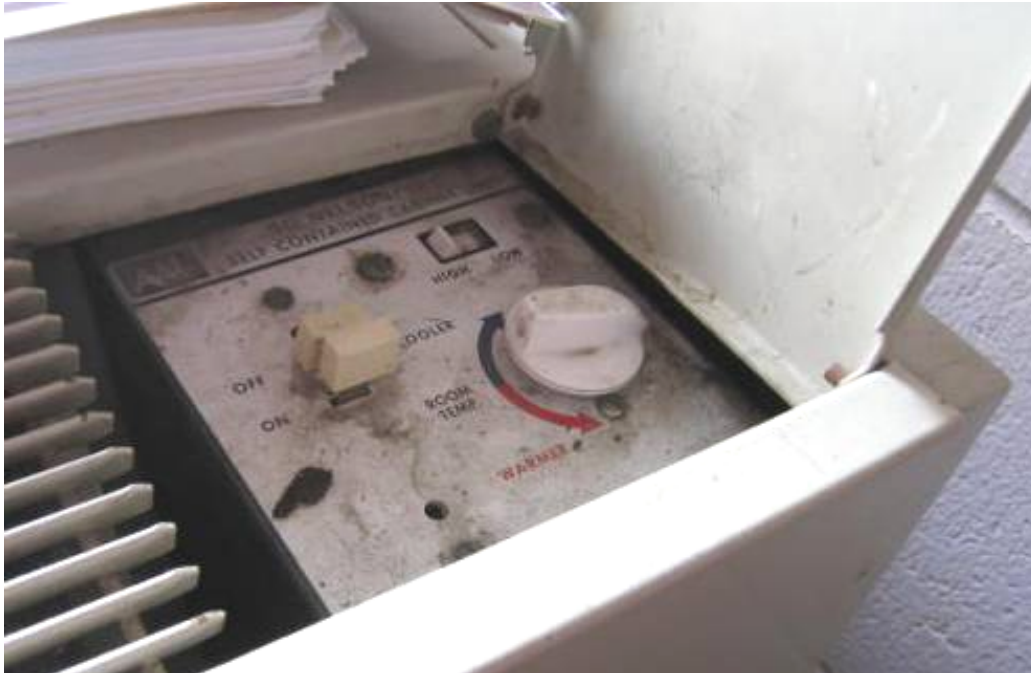
Univent controls, showing unit is shut off
