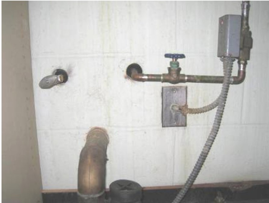
Breaches under sink in room 6A
