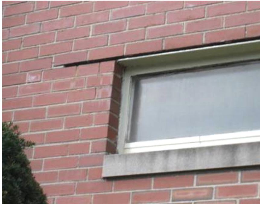
Missing mortar above window
