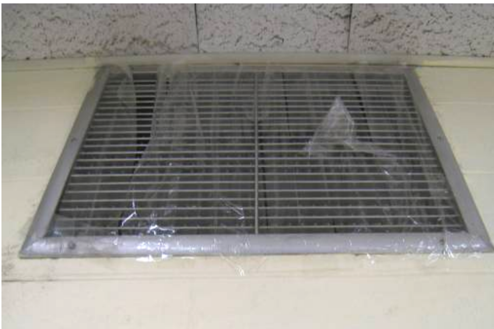
Vent sealed with plastic tape
