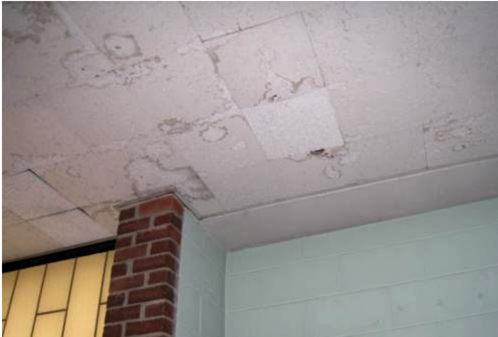
Water-damaged interlocking ceiling tiles
