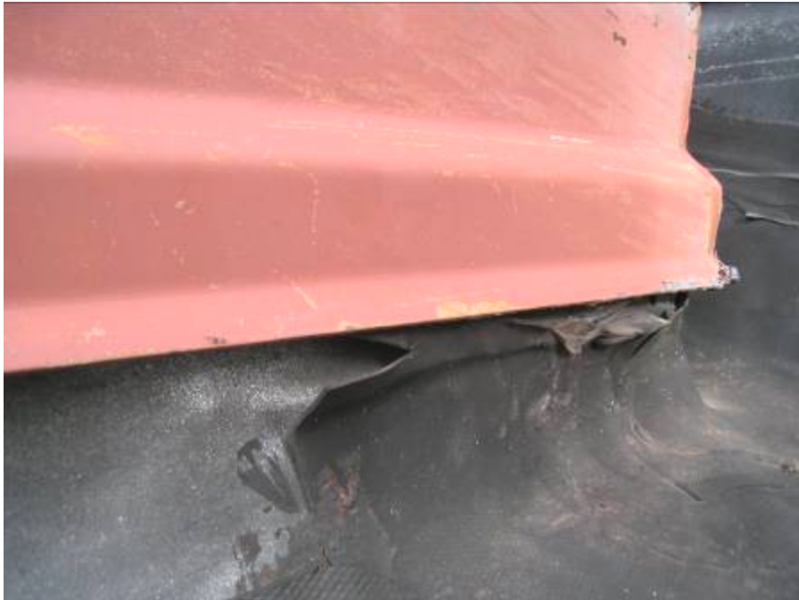
Damaged sealing material around rooftop access hatch
