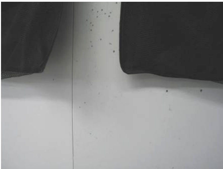
Black staining/possible mold growth on partition wall
