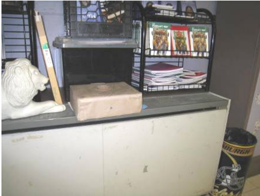
Typical univent, note items on top
