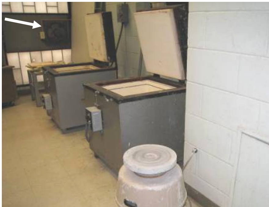
Pottery kilns, note wall-mounted switch-activated exhaust fan several feet away (arrow)
