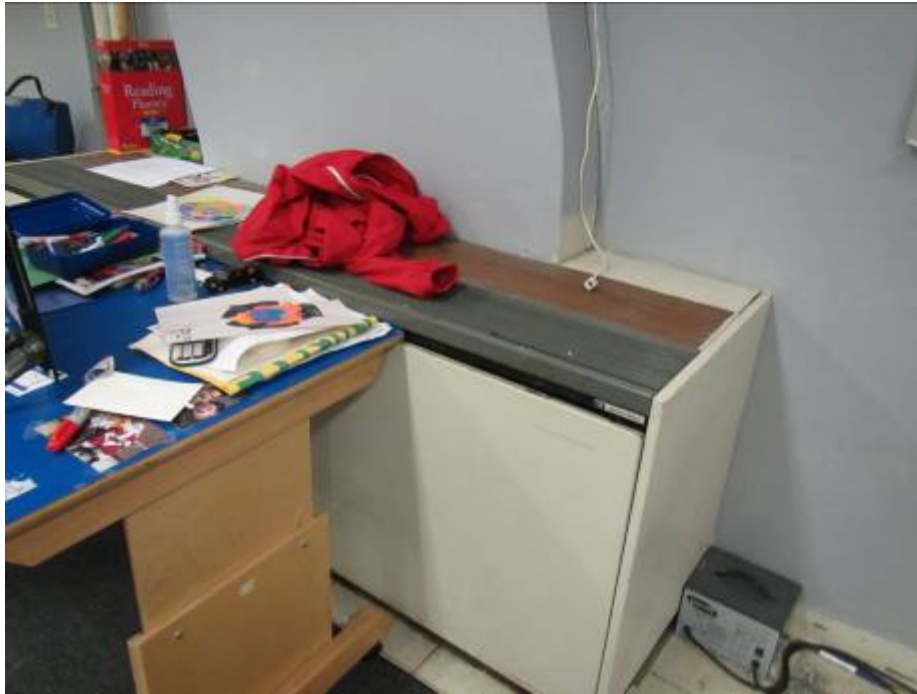
Typical univent, note obstructions, ajar cover, items on top
