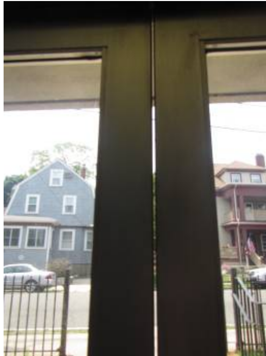
Gaps where doors to outside lack weather stripping
