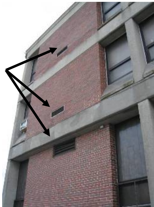
Univent fresh air intakes (arrows)
