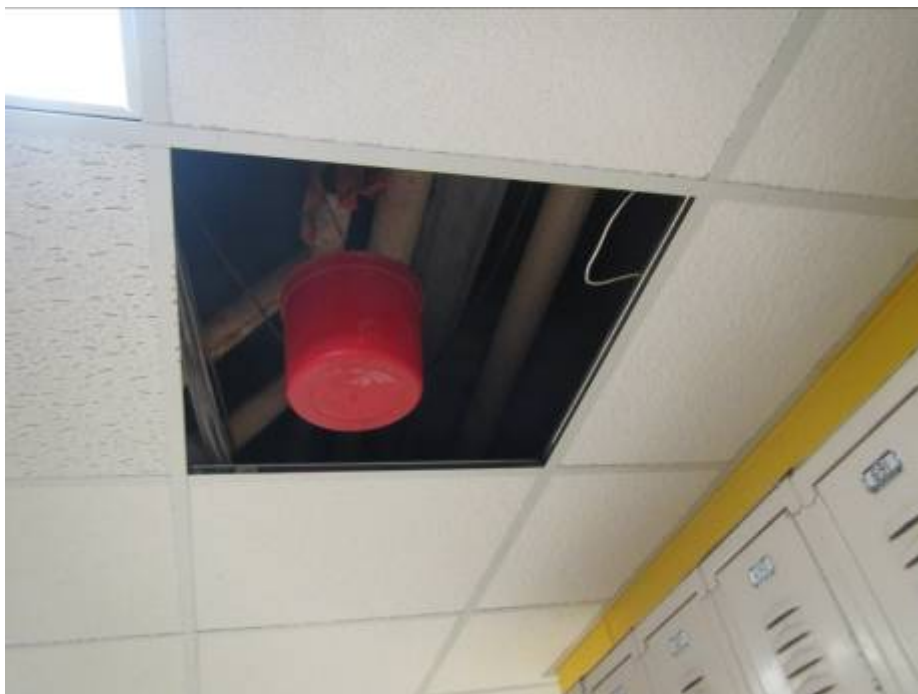
Missing ceiling tile and bucket in hallway
