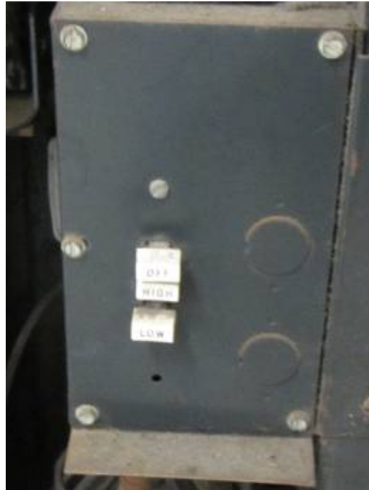
Univent controls, univent is off
