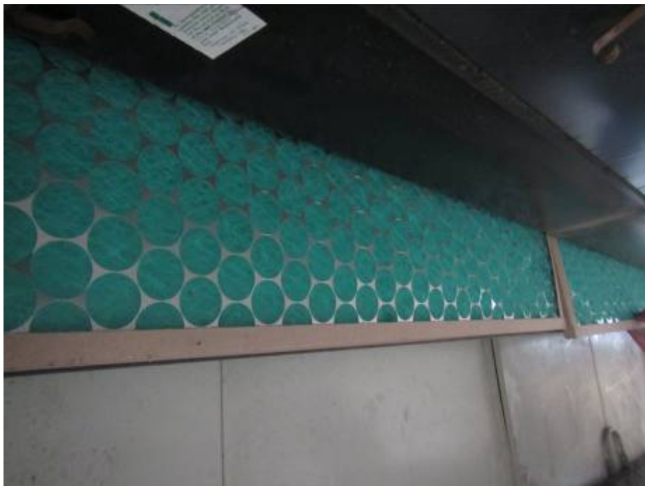
Disposable filter in univent cabinet; this type of filter has a very low dust spot efficiency
