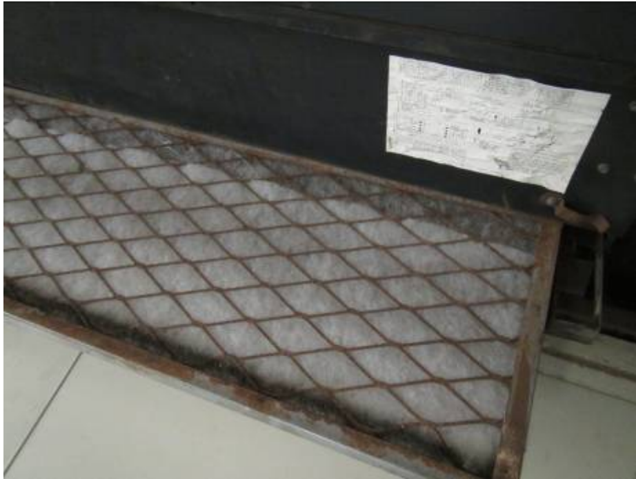
Univent filter medium in lattice cage, note rust/deterioration of cage
