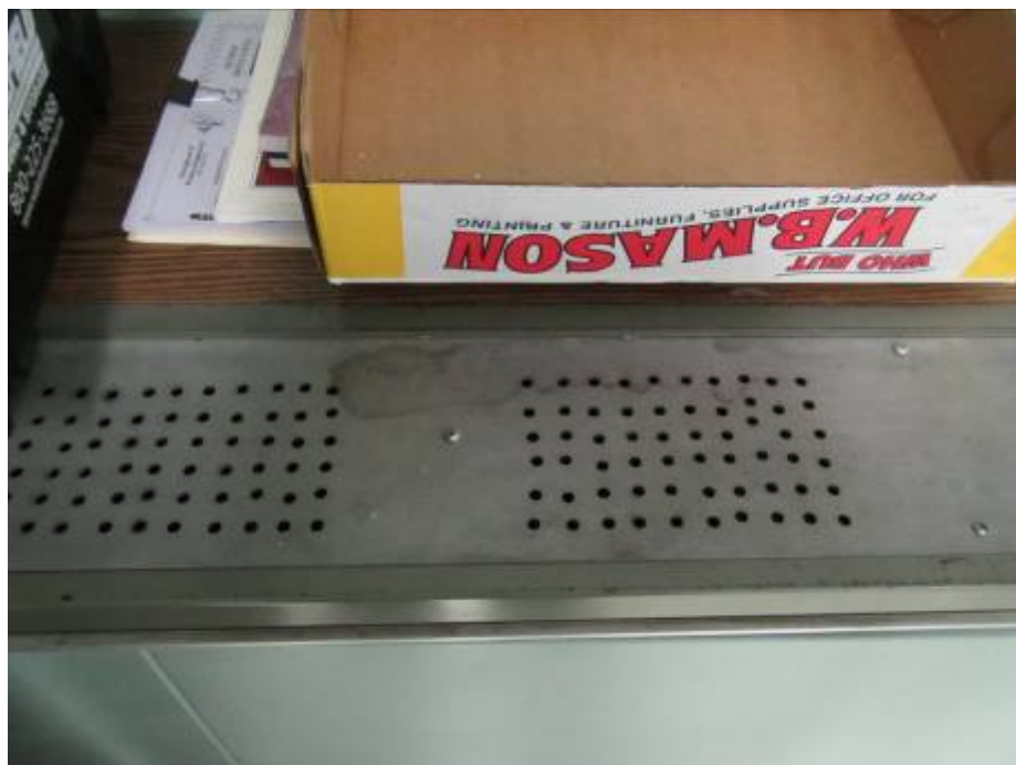
Top of univent showing non-standard replacement diffuser
