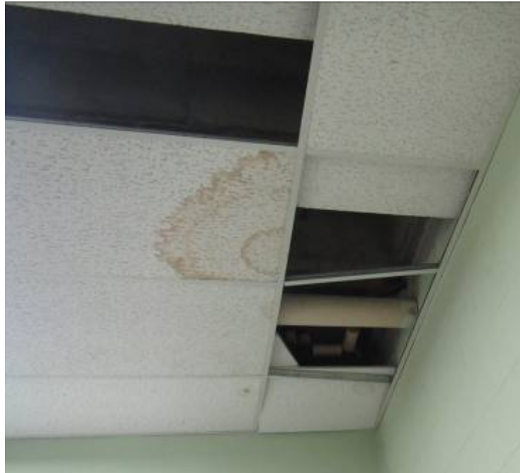
Water-damaged ceiling tiles and missing tiles
